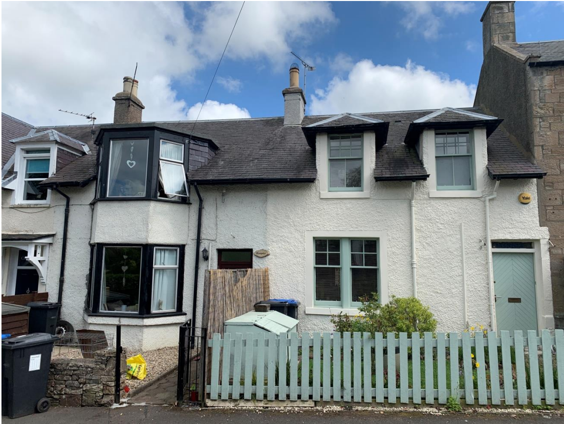
Front Elevation of `Craiglea' & `Glenisla' (Aluminium framed casement to Craiglea, Green painted timber vertical sliding to Glenisla)
